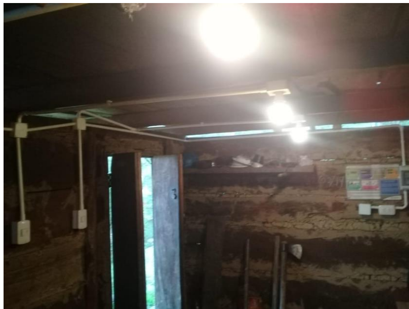
Figure 16 PV system equipment inside casa de campo
