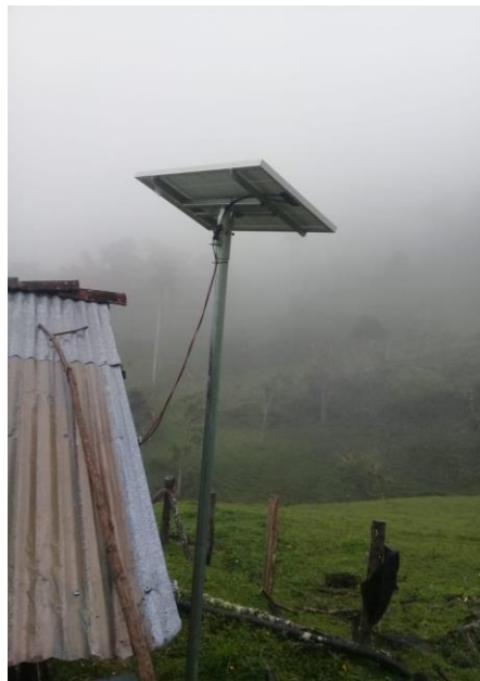
Figure 15 Panel is pole mounted
